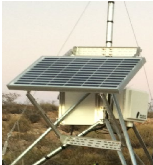
Figure 13—Solar panel mounting
