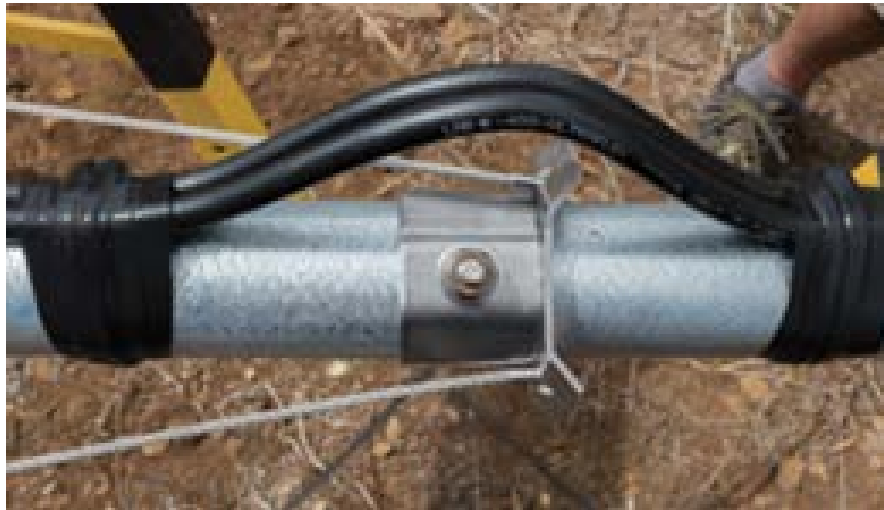
Figure 9—Coaxial cable fed around guy bracket
